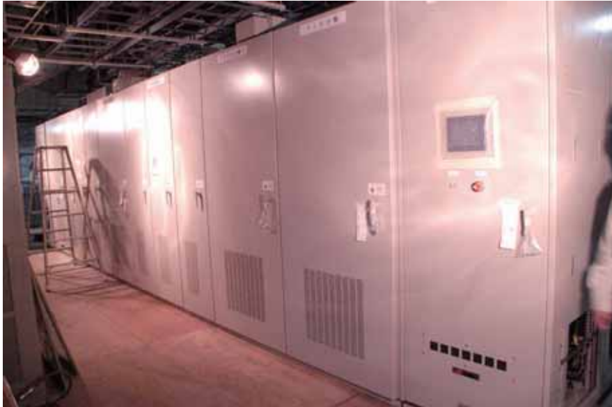
Figure 2 New Magnet Power Supplies for Booster Synchrotron
